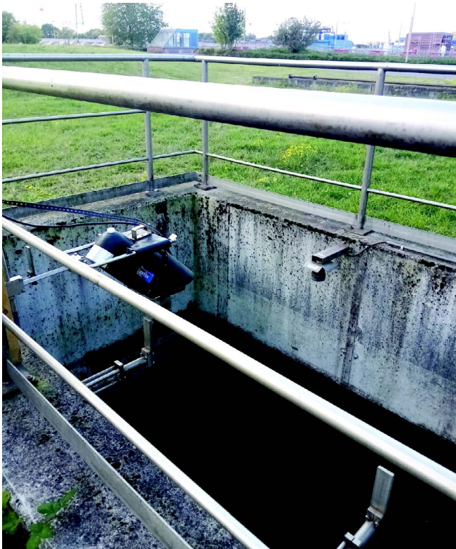
Figure 1: Laserflow At the Final Effluent
