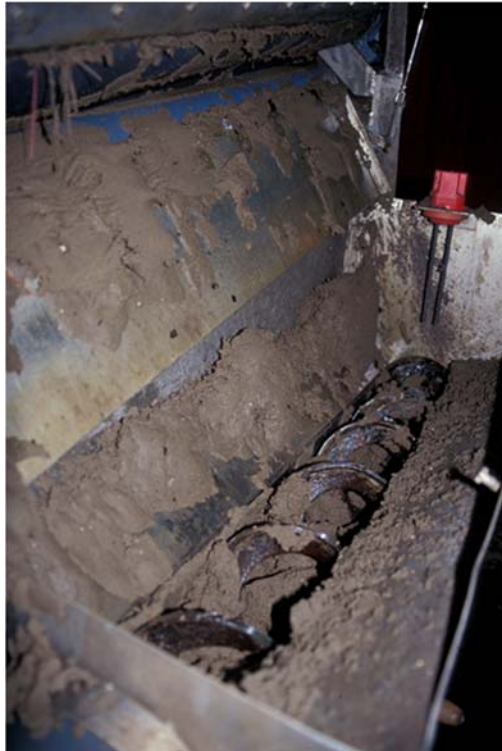
Figure 20. Band filter dewatered sludge outlet.
