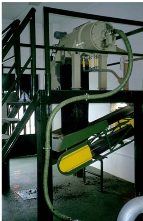
Figure 13. General view of a centrifuge for dewatering.
