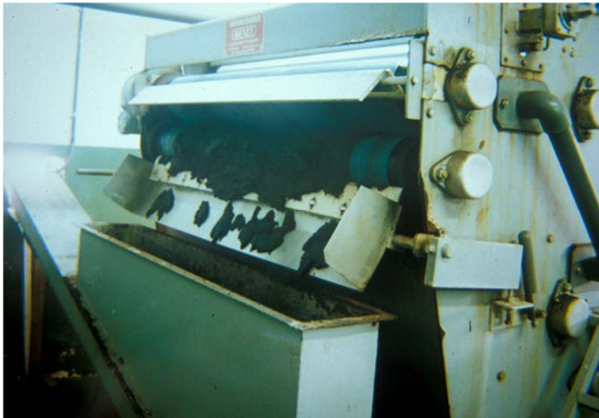
Figure 18. Band filter dewatered sludge outlet.
