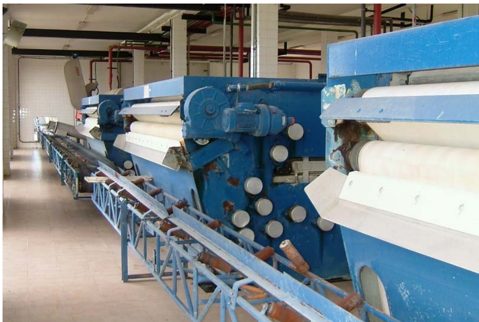
Figure 14. General view of three band filters
