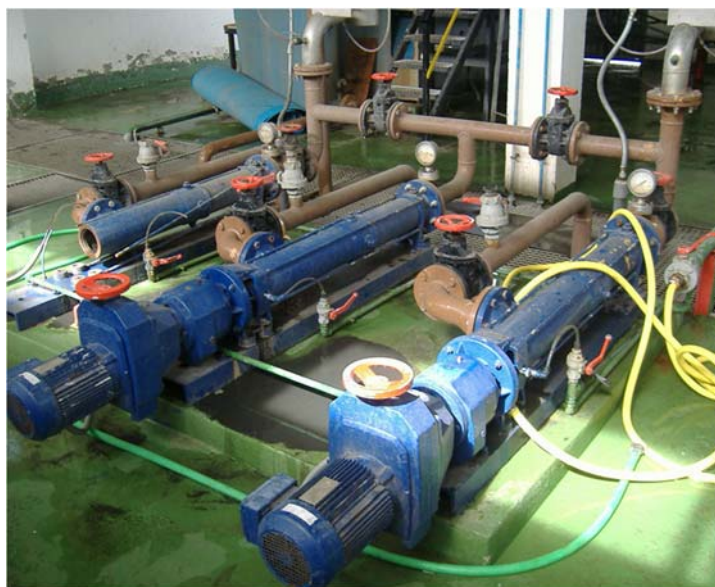
Figure 1. Positive displacement pumps for sludge conveying.
