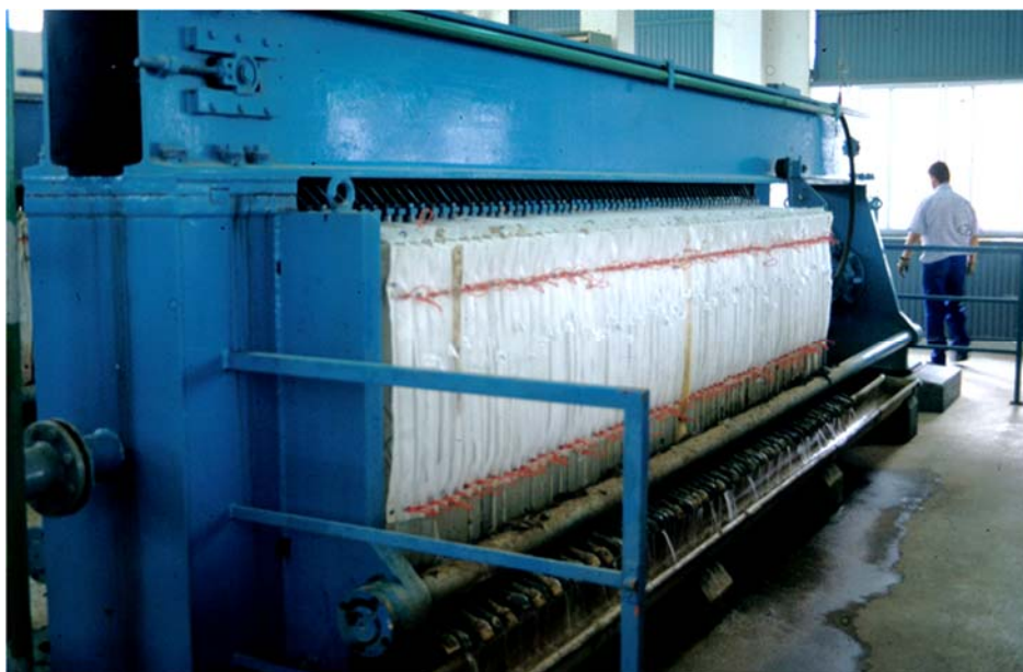
Figure 23. General view of a press filter in operation (Santiago de Compostela).
