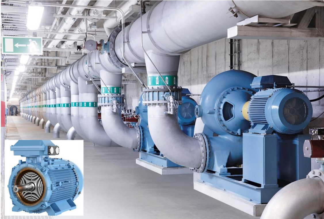
Figure 21 Pumping station using Synchronous Reluctance Motors (source:ABB)
