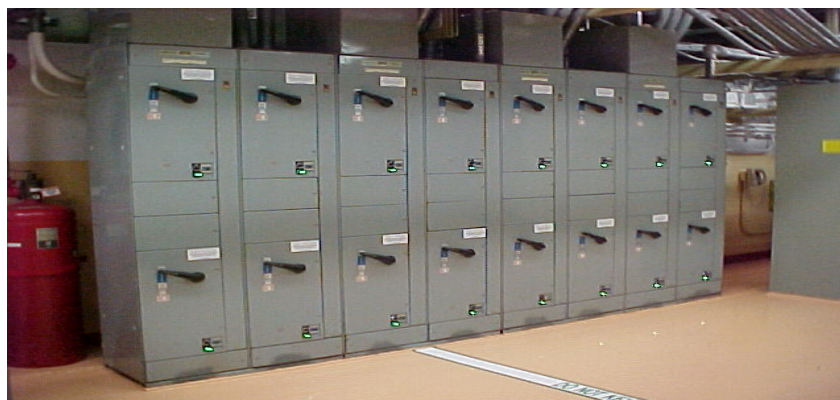
Figure 6: Example of Motor Control Center (MCC)
