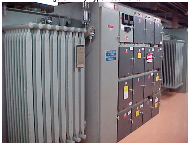
Figure 5: Liquid-Cooled Load Center
