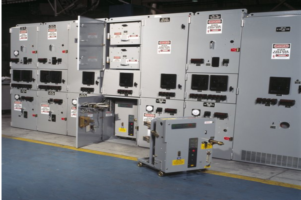
Figure 2: Medium Voltage Switchgear
