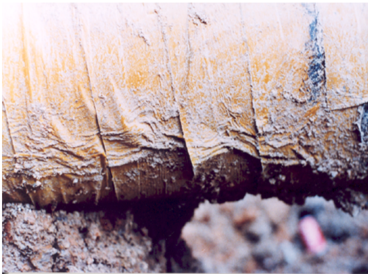
Figure 9-3. Disbonded solid film-backed tape coating.
