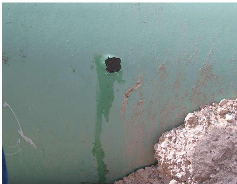
Figure 9-1. Water under blister on FBE coated pipeline. No corrosion under the blister and water had a pH of 12 indicating that CP was able to protect under the disbonded, non-shielding FBE.
