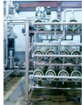
Membrane filtration plant
