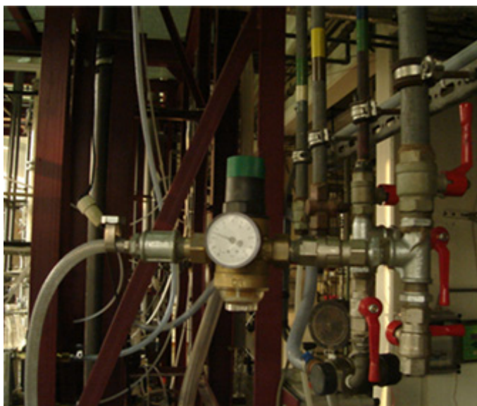
FIGURE 3.5. DETAIL OF MANOMETER TO CONTROL PRESSURE IN TAP WATER FLOW
