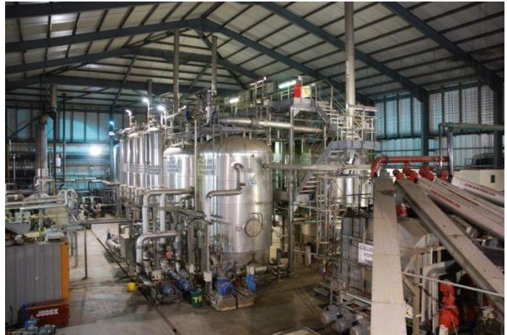
Thermal hydrolysis (CAMBI process): Ringsend WWTP Dublin (Ireland)
