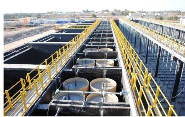
Figure 5: TURBO4BIO Installation at Kufa
