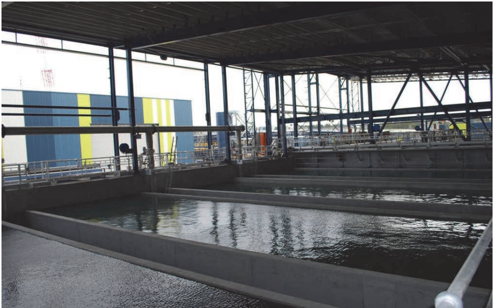
Fig. 25. Gravity dual media filters (Australian desalination plant)
