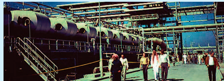
Figure 13. A single MSF unit at Al-Jubail Phase 2
