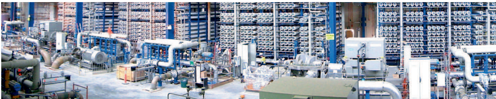
Figure 17. A typical large SWRO plant
