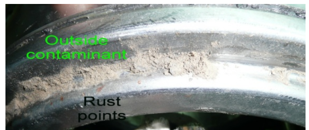
Corrosion. Contaminant deposit.
