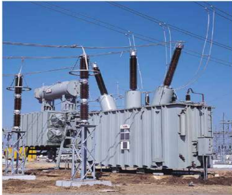
100 MVA, 220 / 66 kV Power Transformer
