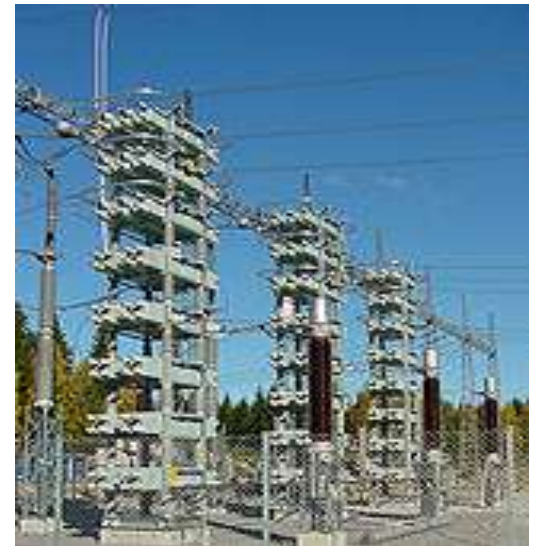
400 Mvar shunt bank for reactive compensation
