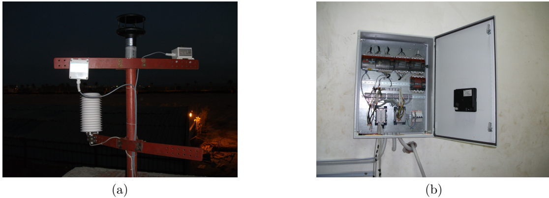
Fig. 5.11.: a) Weather station with different sensors at the roof. b) Switch cabinet with the Trend controller and the touch screen in the building.
