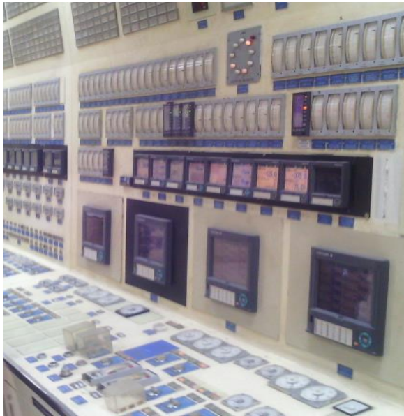
Old look of Conventional Control Room, Where every instrument installed on the Desk & panel
