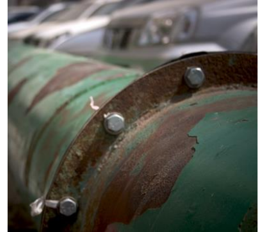
Poor adherence of the paint
