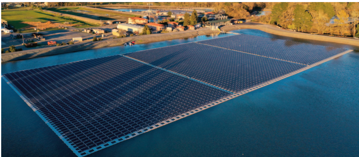
Floating PV site in Windsor.
