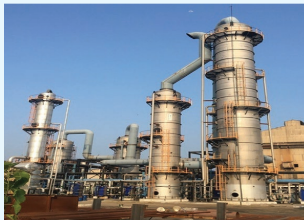
Figure 3-3: CO 2 Capture Plant at Tuticorin Alkali & Chemicals
