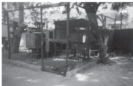
Fig. B26 : Outdoor substations without enclosures
