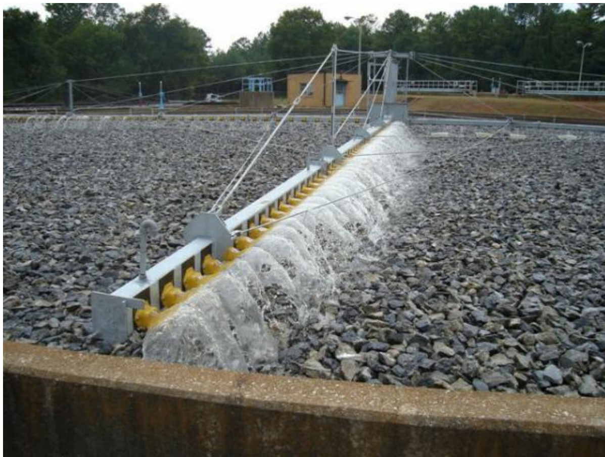
Figure 4-7 Photographic view of rotary distributors
