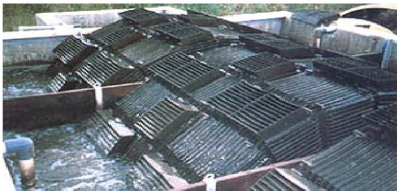
Figure 4-19: Rotating Biological Contractors placed in series
