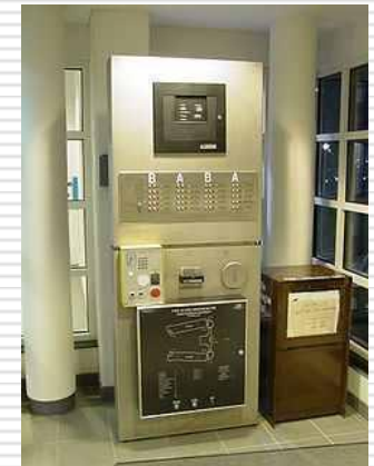
An integrated control panel
