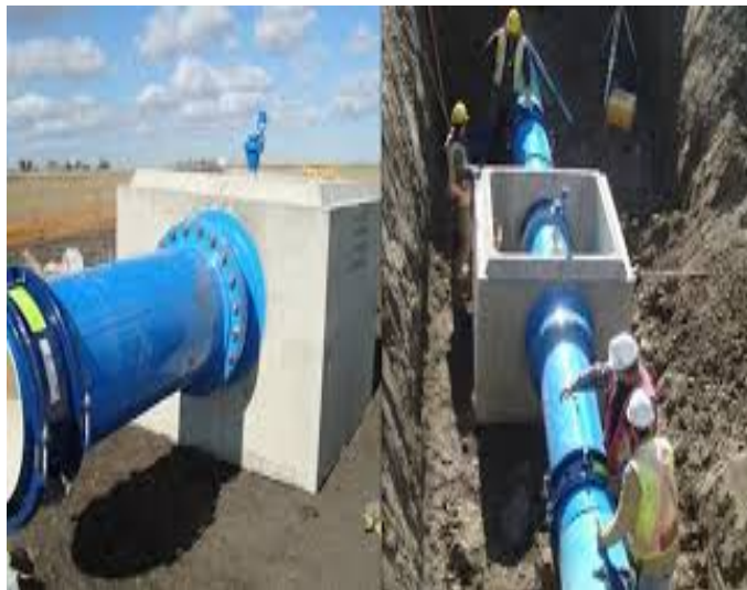
AIR VALVE CHAMBER
