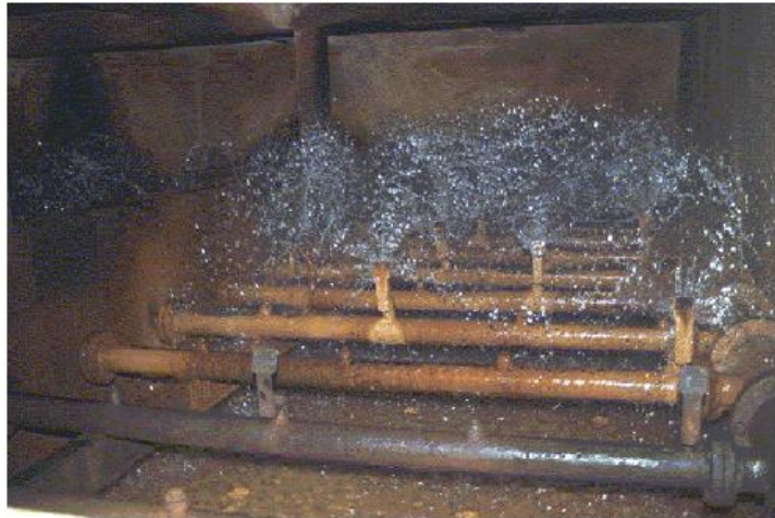
Figure 4 - Aeration above limestone filter
