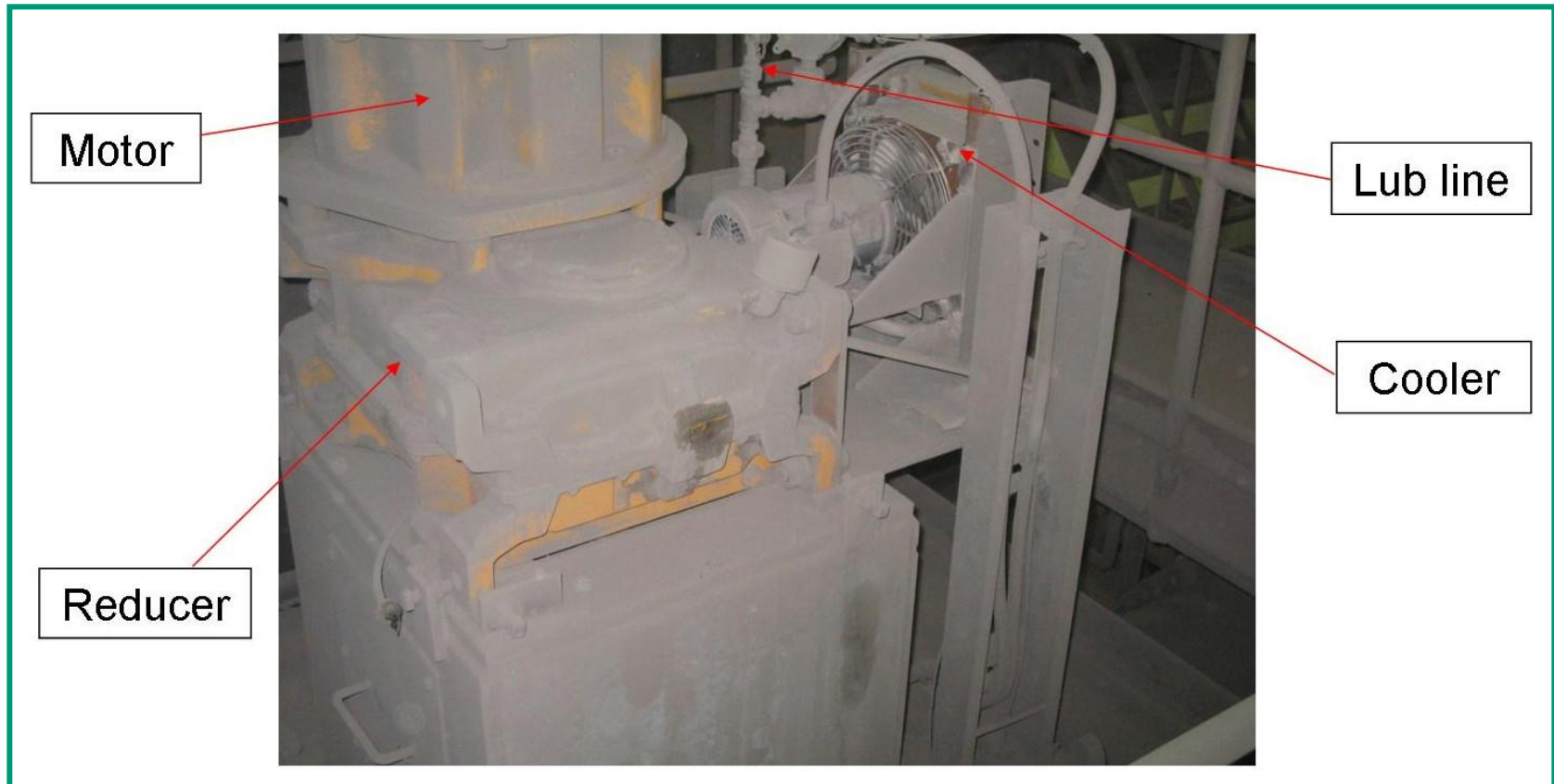
Reducer with circulating system. Oil pump located underneath of the reducer.
