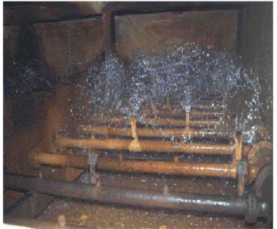
Figure 4 - Aeration above limestone filter
