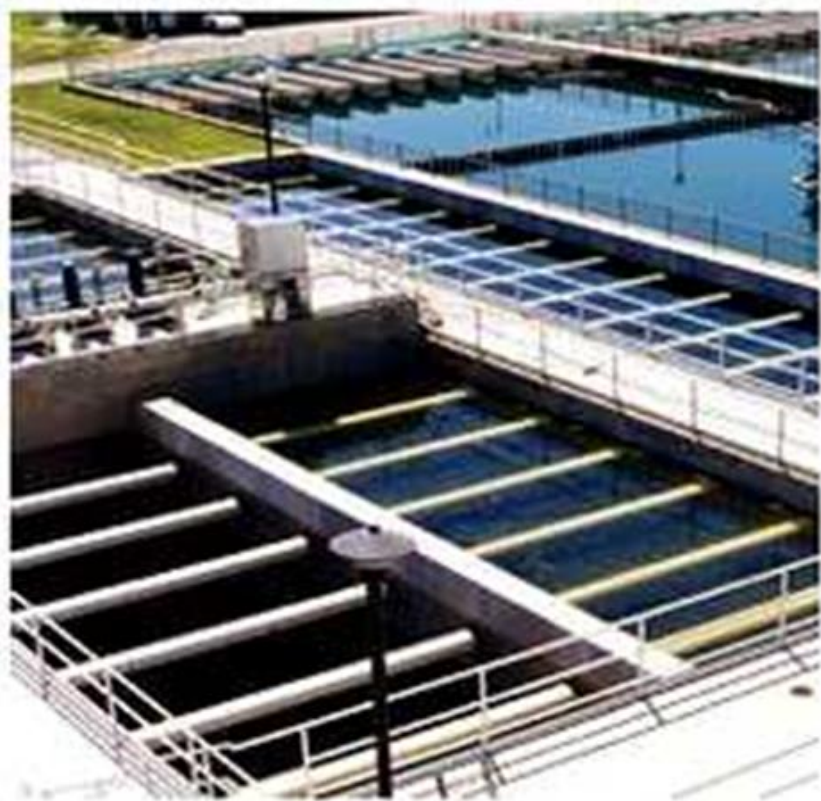
Super-Pulsator Flocculator Clarifiers in operation.
