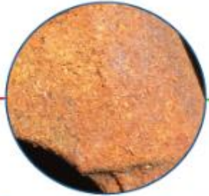
General (or Uniform) Corrosion
