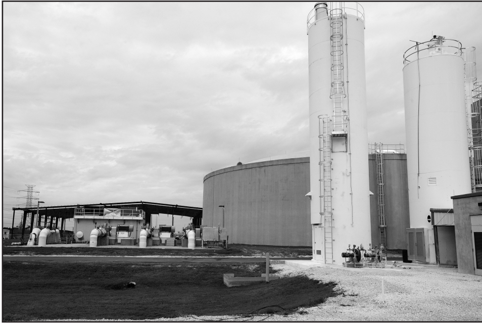
Figure 8-1 Water treatment plant
