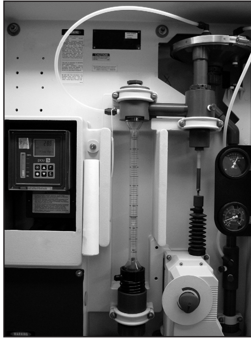
Figure 8-4 Chemical feed system, a gas chlorinator ( Opflow 2010 )
