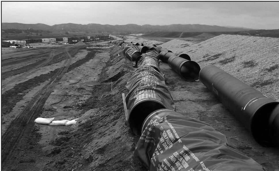
Figure I-1 Large water transmission pipeline (courtesy of Beaumont Cherry Valley Water District, J. Reichenberger, P.E., District Engineer)
