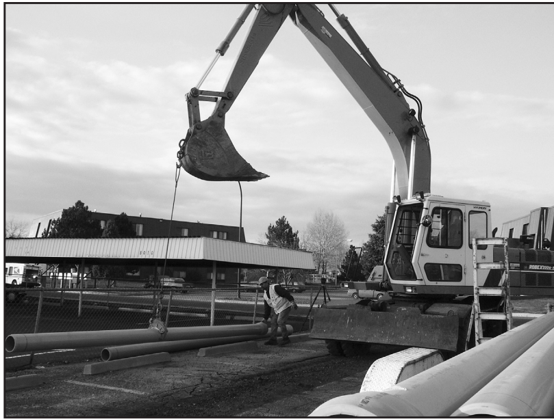
Figure 11-3 Pipe storage can present problems
