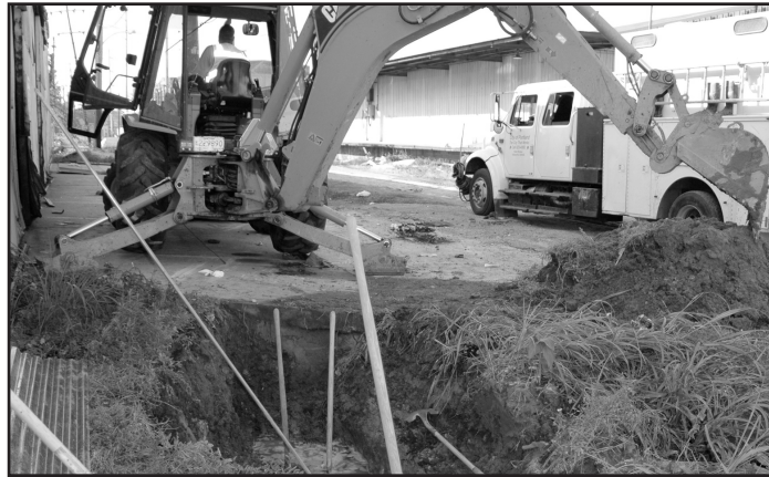
Figure 2-2 Repairs after Hurricane Katrina
