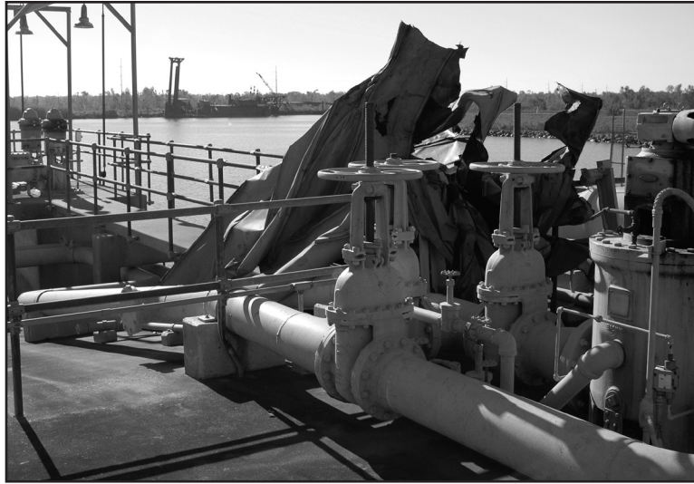
Figure 2-1 Damage from Hurricane Katrina
