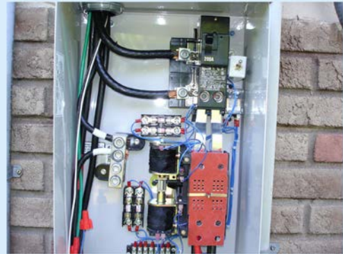
Standby System Capacity - Automatic Transfer Equipment 702.4(B)(2)(a)
