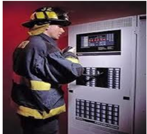
Figure 239: Fire alarm control units
