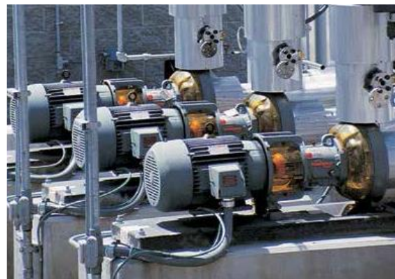
Figure 103: RO pumps and instrumentation
