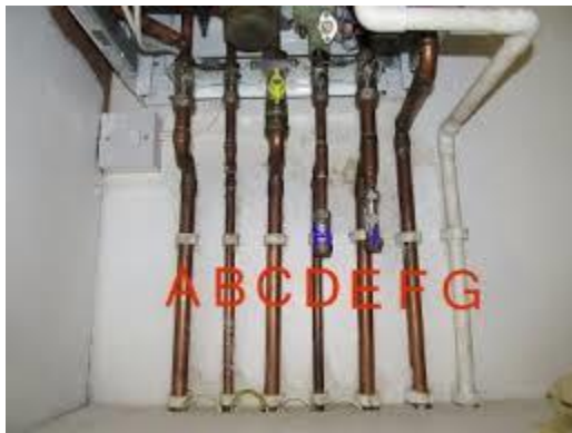
Figure 128: Condensate pipe works
