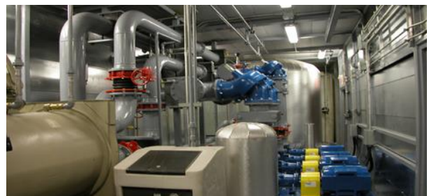
Figure 170: Piping and Valves
