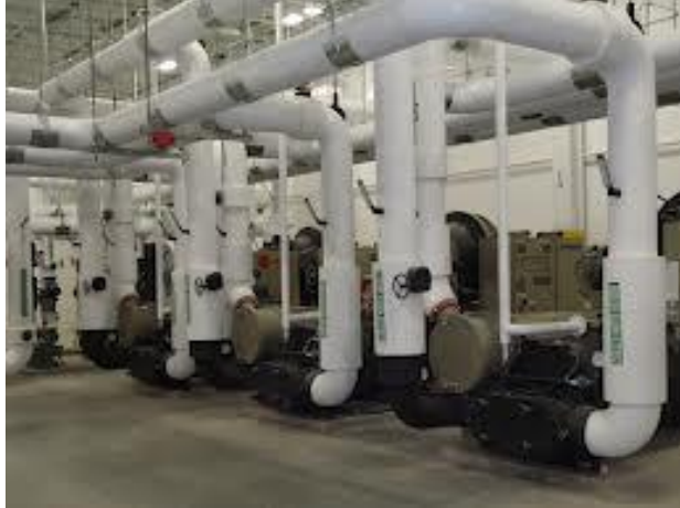
Figure 127: HVAC piping and pumps
