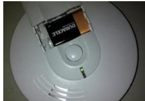
Figure 241: fire alarm Battery
