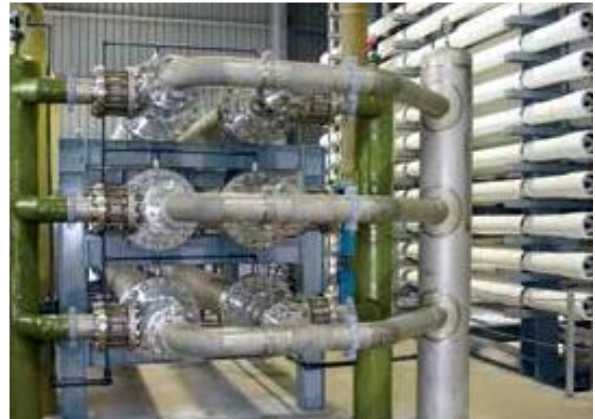
Figure 104: RO plant pipe works
