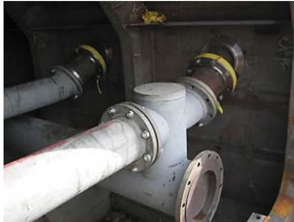
Figure 3.8: Flange Joints on Pipeline
