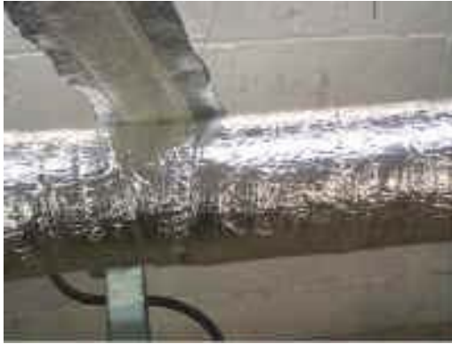
(a) Silver Layer Next to Pipe
