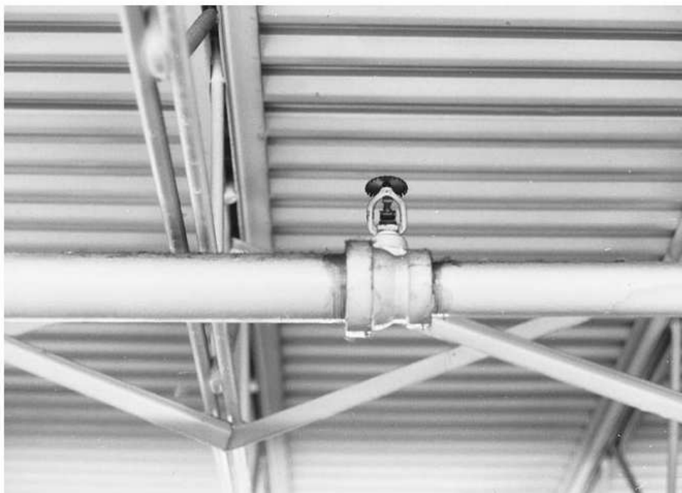
Photo 2 An installed brass upright sprinkler head. This sprinkler should not have been painted!
