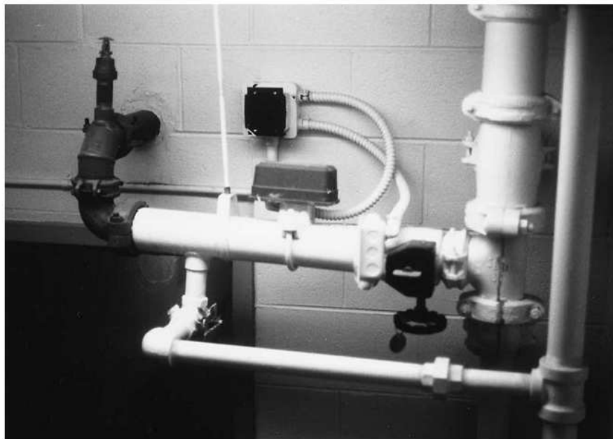
Photo 9 Located near the ceiling, this system cut-in to a combination standpipe includes a butterfly valve, flow switch, and a system drain that is piped to an express drain. Note that the drain valve is correctly placed downstream of the flow switch.
