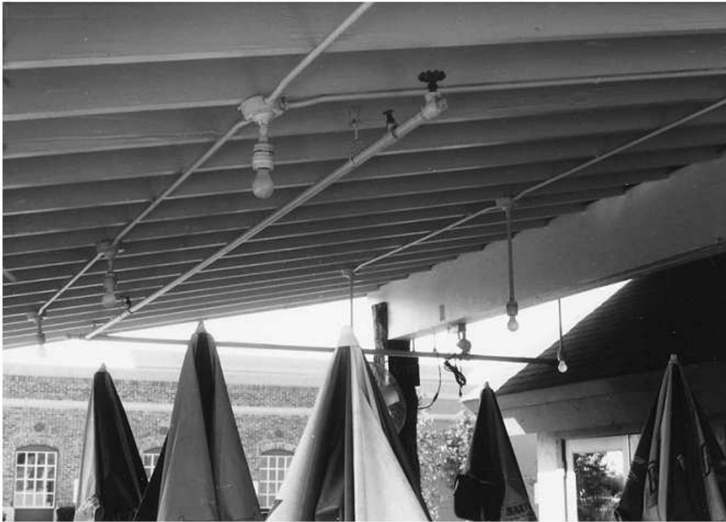
Photo 6 These sprinklers installed beneath a combustible outdoor roof section are part of an anti-freeze system.
