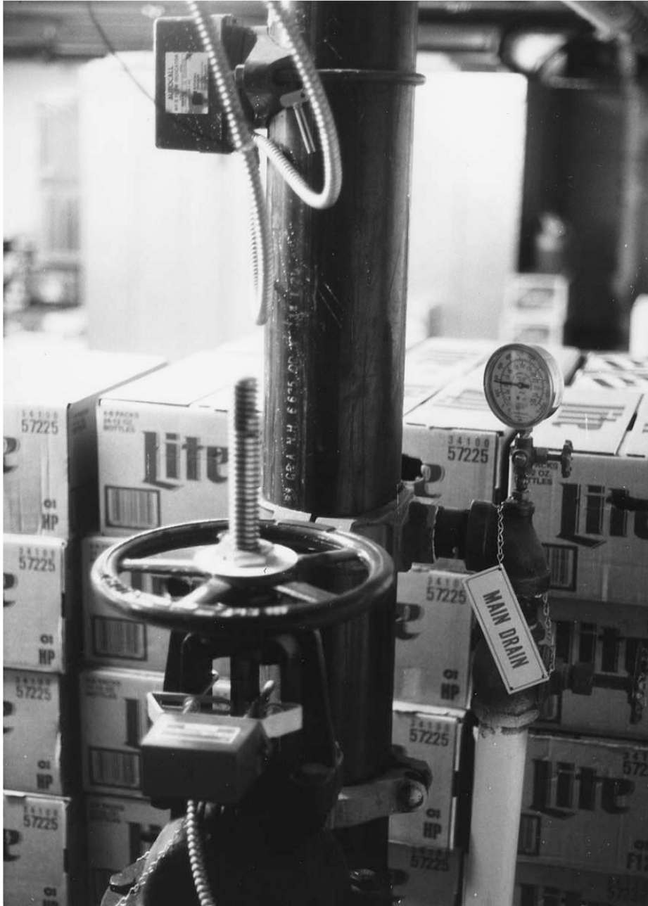
Photo 14 This shows an acceptable pressure gauge installation, which has been piped off of the riser on the 2" main drain piping upstream of the drain valve.
