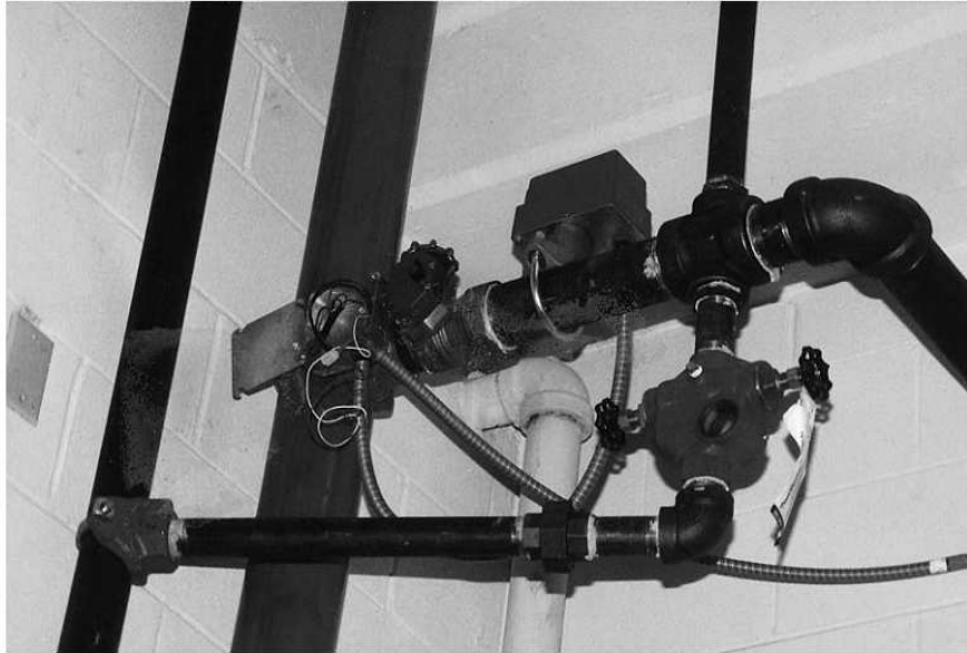
Photo 10 Another system cut-in made on a combination standpipe in a high-rise building. The component shown downstream of the flow switch is a combination system drain/inspector's test connection.
