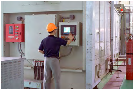
Figure 10.3 Typical on-skid control
