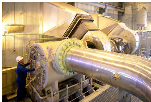
Figure 3.6 Titan 130 compressor set
