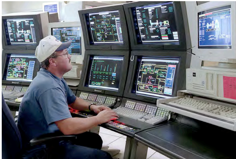
Figure 5.4 Compressor test facility control room
