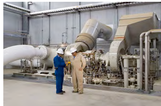
Figure 3.5 Centaur 50 compressor set
