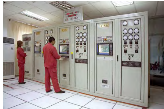
Figure 10.4 Typical control room
