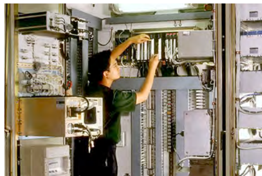
Figure 10.5 Control console interior components
