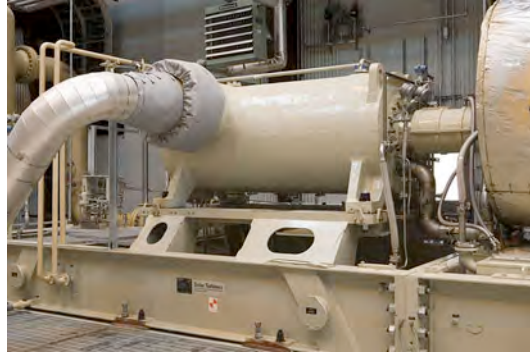
Figure 1.6 C51 production compressor
