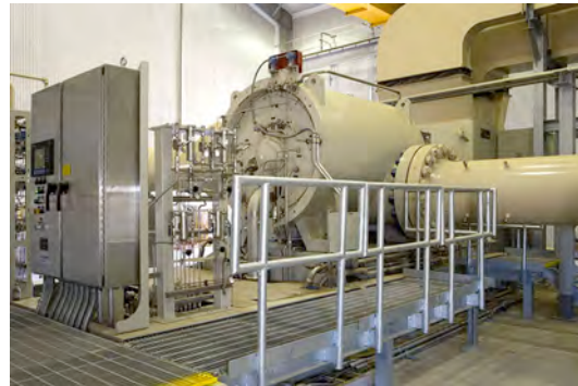
Figure 1.4 C65 pipeline compressor
