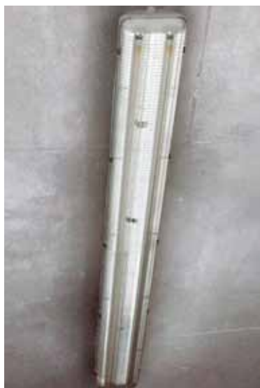
Artificial lighting with unbreakable cover
