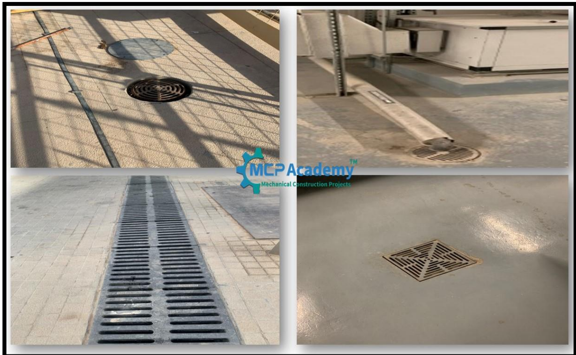
Roof Drain, Floor Drain, Channel Drain and Area Drain (PHOTO FROM SITE)
