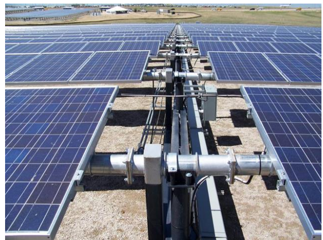
Figure 40: Active Sun-Tracking Arrays Use Hydraulic Pistons, Pneumatic Pistons or Motors to Drive the Tracking Mechanism for Single Rows or Multiple Subarrays
