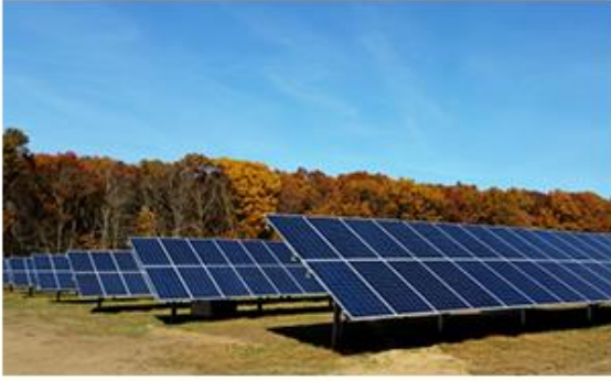
Eau Claire Energy Cooperative - 750 kW AC
