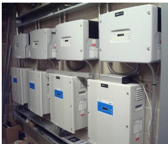
Figure 33: String Inverters Use Series-Connected Array Designs
