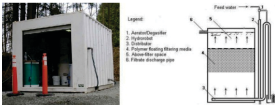
Figure 67: Iron Stopper Containerized Treatment System
