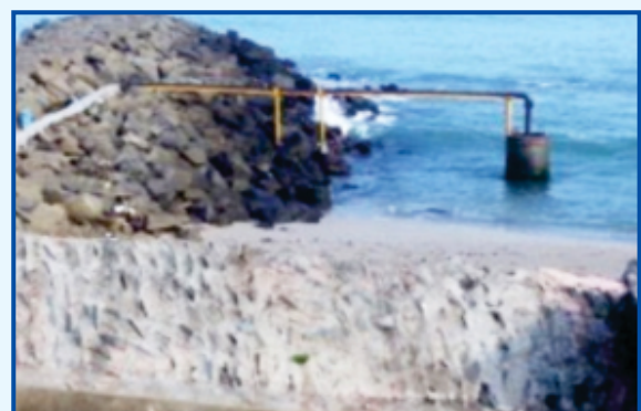
d. A view of the Sea water intake system
