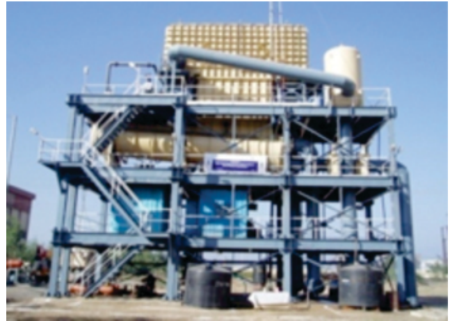
Figure 81 : View of the Commissioned LTTD Plant at NCTPS
