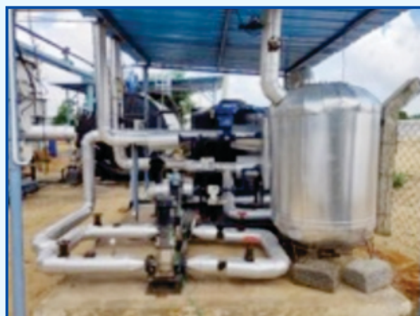
Solar hot water system installed
