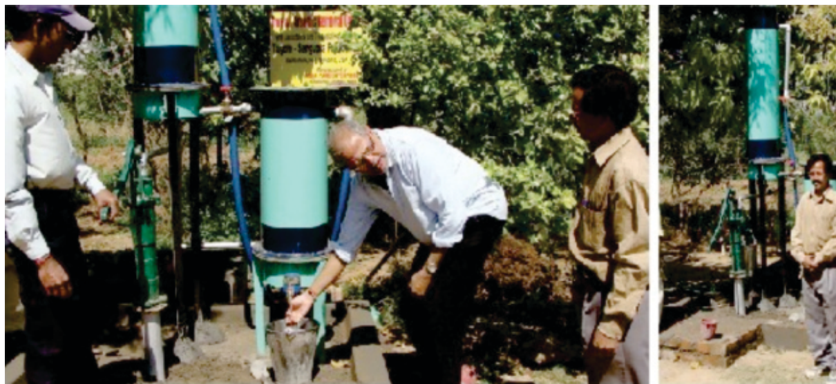
Figure 34: Arsenic Removal Plant at Rampur - Maner
