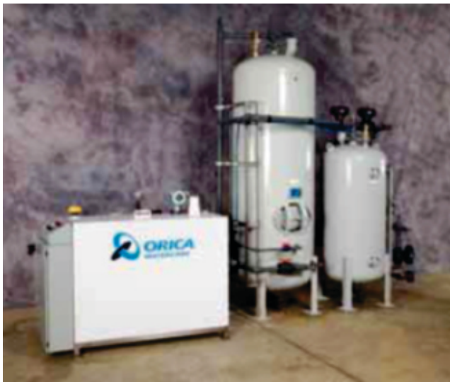
Figure 72: MIEX Treatment Systems
