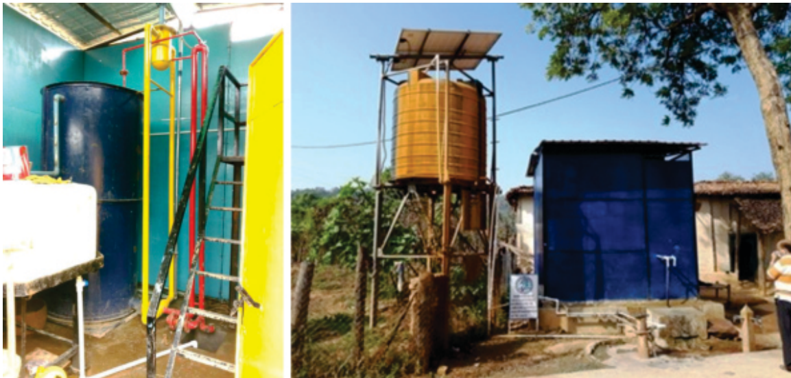
Figure 68: Self-Sustained Auto Backwash Iron Removal Plant
