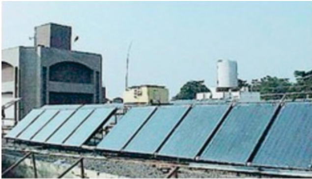
Figure 88.2: Flat-plate-collector-based solar desalination system installed at the SEC, Gual Pahari, Gurgaon
