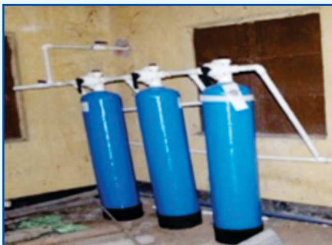
Treatment unit within room in the school
