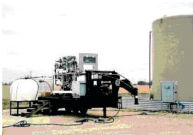
Figure 91: A&M Mobile Desalination Unit
