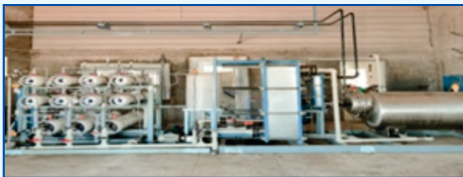
Forward Osmosis system installed at Narippaiyur Village
