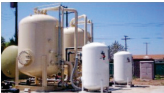
Figure 73: Siemens Nitrate Removal System
