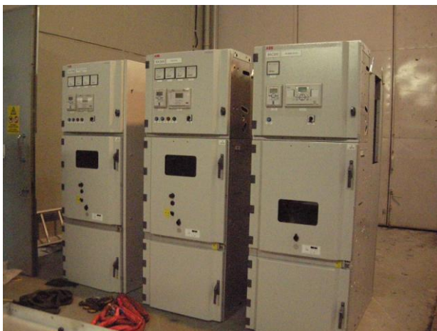
Picture 2, Switchgear cabinets
