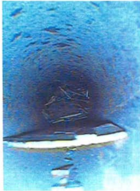
Internal blockage in a lower loop from exfoliation.
