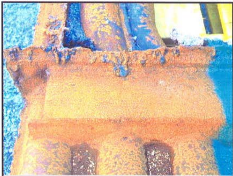
This shows a seal box on the cold side of waterwall tubes. They are restrained by this box and have failed due to corrosion fatigue
