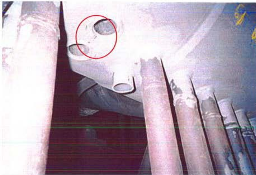
Figure 1. Tube location 63 of Unit #4 high-temperature reheat header (HRH) that experienced ligament cracking.
