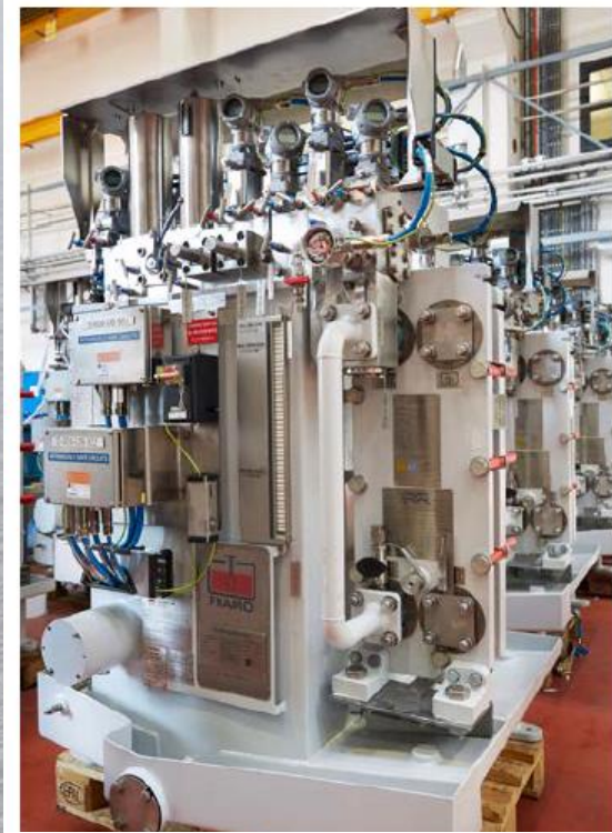
Lube oil circulation unit (OCU) Sergio Vidal
