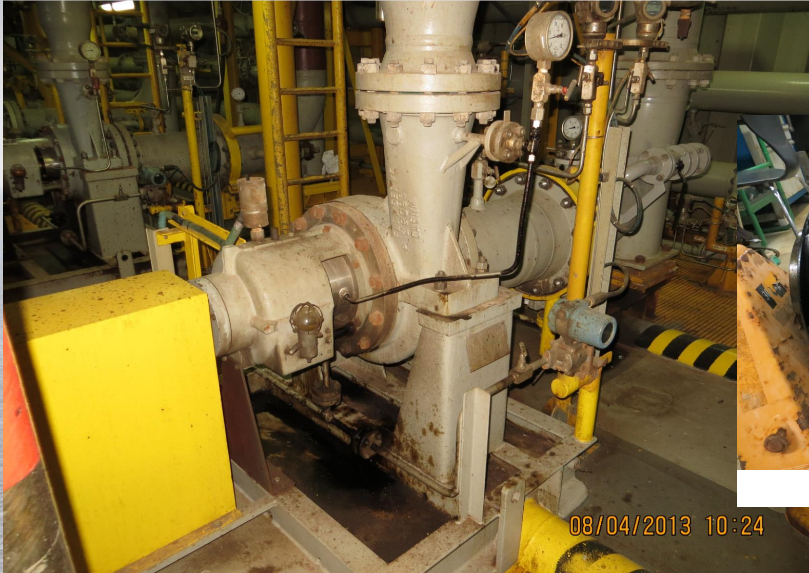
API OH2 Crude oil export pump picture
