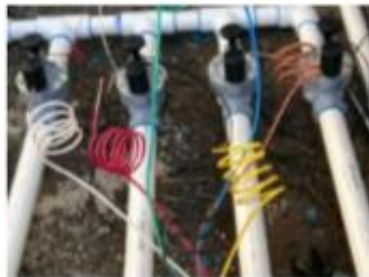
Wires at Valves
