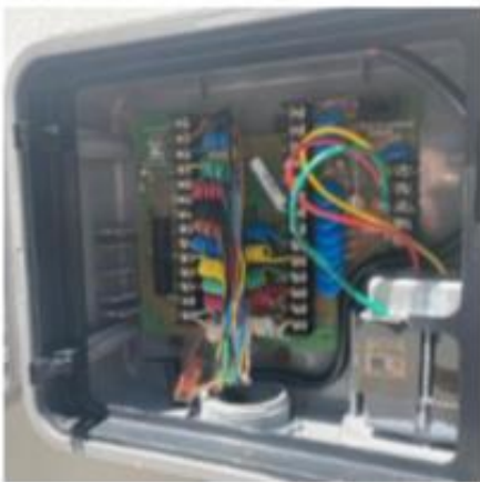
Wires at Controller
