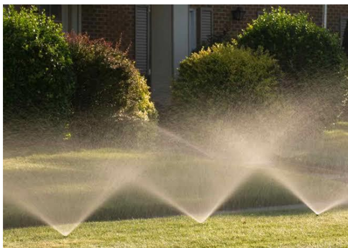
Pop-up sprinklers and Spray Heads for Lawns
