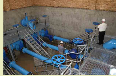
Figure 11: Sebokeng/Evaton pressure management installation
