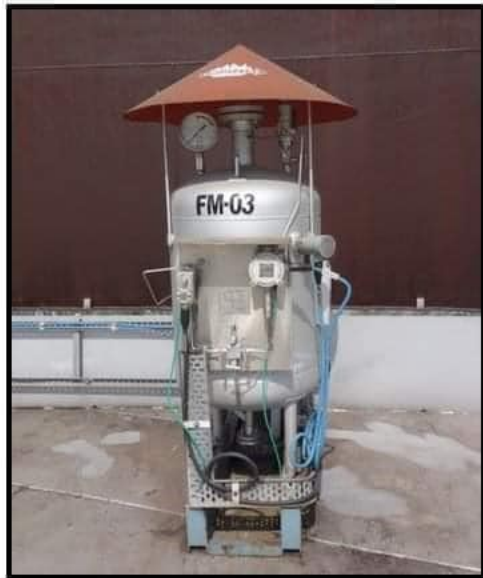
Rim seal fire protection
