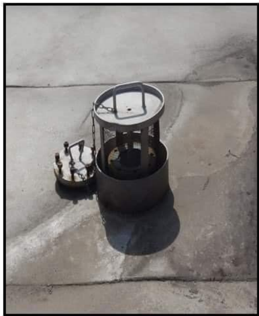
Emergency Roof drain
