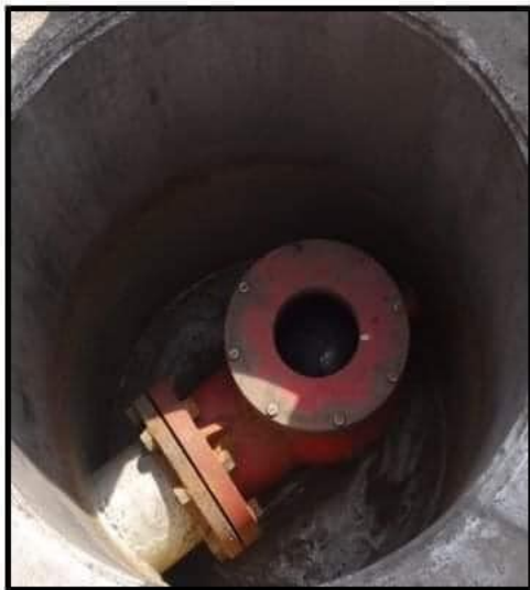
Roof Drain- NRV
