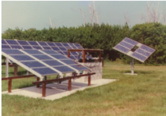
Rack and Pole mounted Arrays
