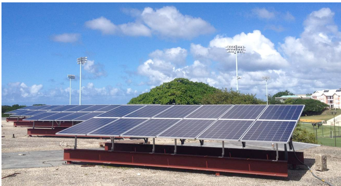
A 12kWp PV system donated to the Cave Hill campus by the Government's Energy Division
