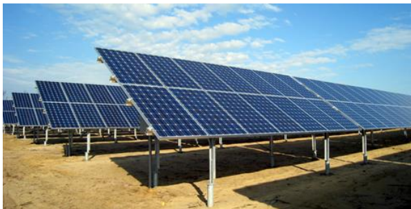
Figure 8 – Ground mounted PV array
