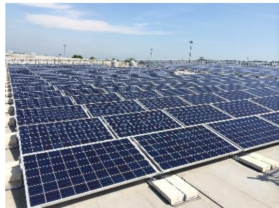
Figure 9 – Rows of PV modules on rooftop
