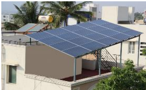
Figure 12 – Canopy on rooftop (BAPV)
