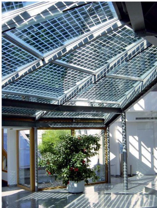
Figure 10 – PV on inclined rooftop (BIPV)
