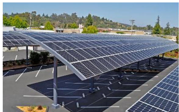
Figure 17 – PV canopy (BIPV)
