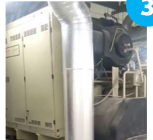
Seawater-cooled, oil-free chiller system
