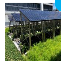
Solar PV system
