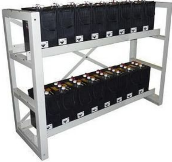
Stationary batteries on a rack (courtesy of Power Battery)
