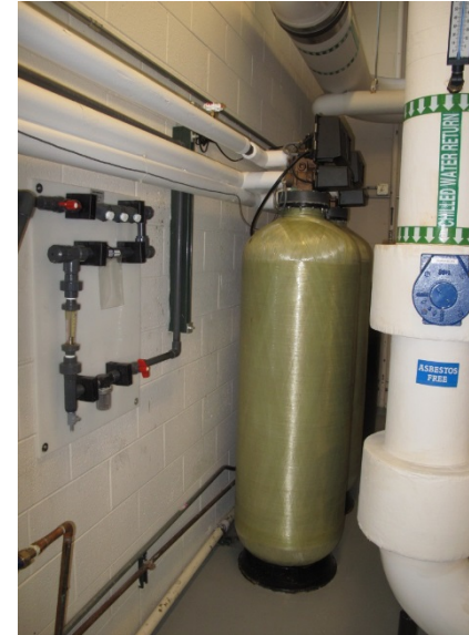
AWT #2 Regeneration and Brine Tank
