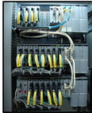
Figure 15: Link Between Master Rack and Extension Racks
